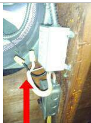
Improper electrical connection at exhaust fan. Have electrician repair.
