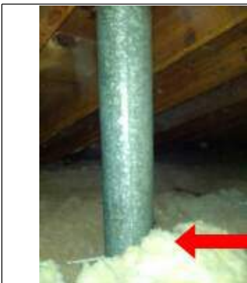
Insulation contacting chimney flue is a fire hazard. Requires at least 2 inch clearance from combustibles.
