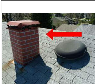
Chimney height is marginal. Recommend extending to a minimum of 2 feet above the roof ridge.
