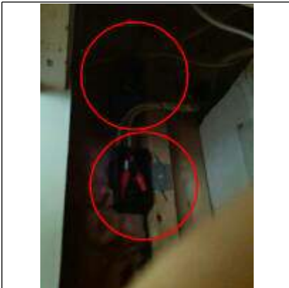
Open junction boxes, safety hazard, recommend covers
