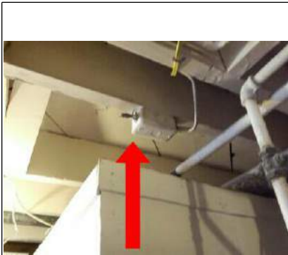
Exposed cut wire. Recommend electrician remove.
